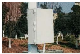
Fixed on the telegraph pole
